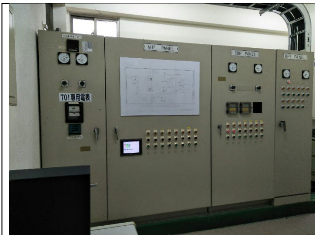
Sewage plant central control room
