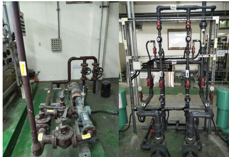
Sewage plant treatment equipment
