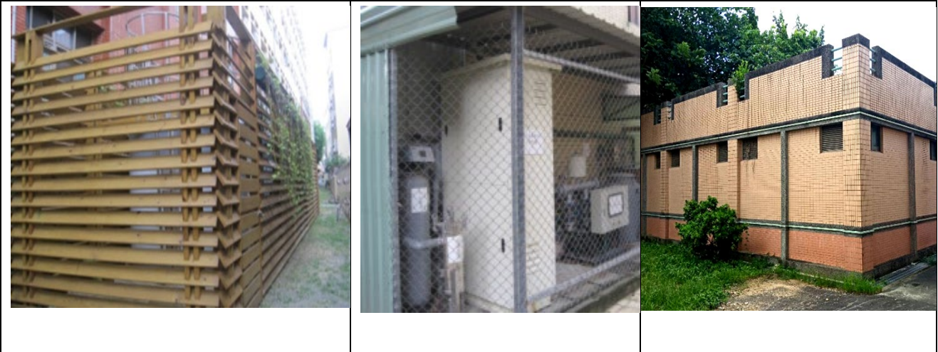
Guoxiu Teaching Building Rainwater Recovery System, NCUT
